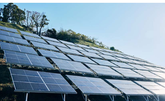
Solar panels on the factory grounds
