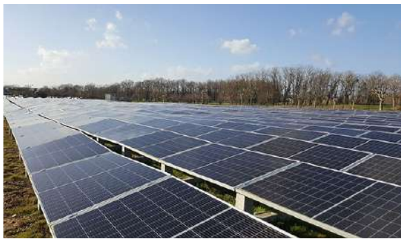
Solar panels at the Gien factory (France)
