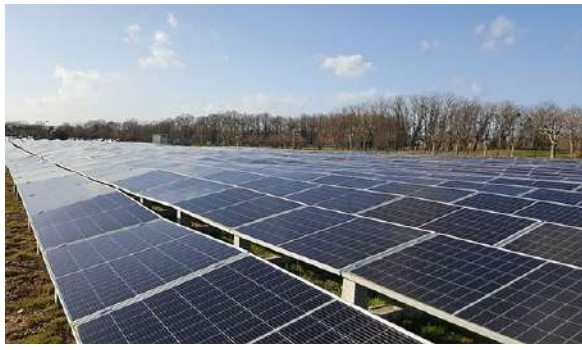
Solar panels at the Gien factory (France)
