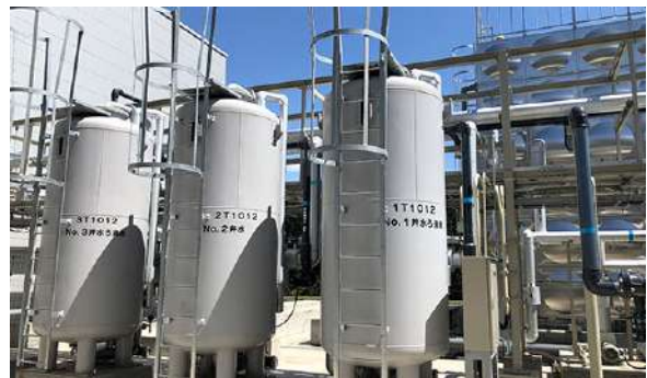
Groundwater purification system at the Nasu Factory (Japan)
