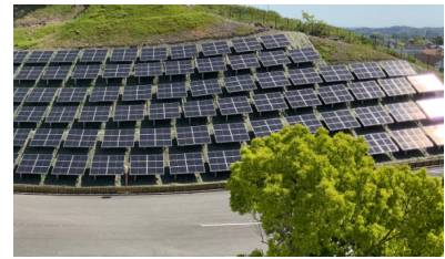
Solar panels at the Kakegawa factory (Japan)
