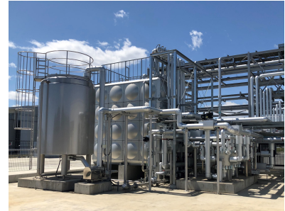
Water saving equipment at the Nasu factory (Japan)
